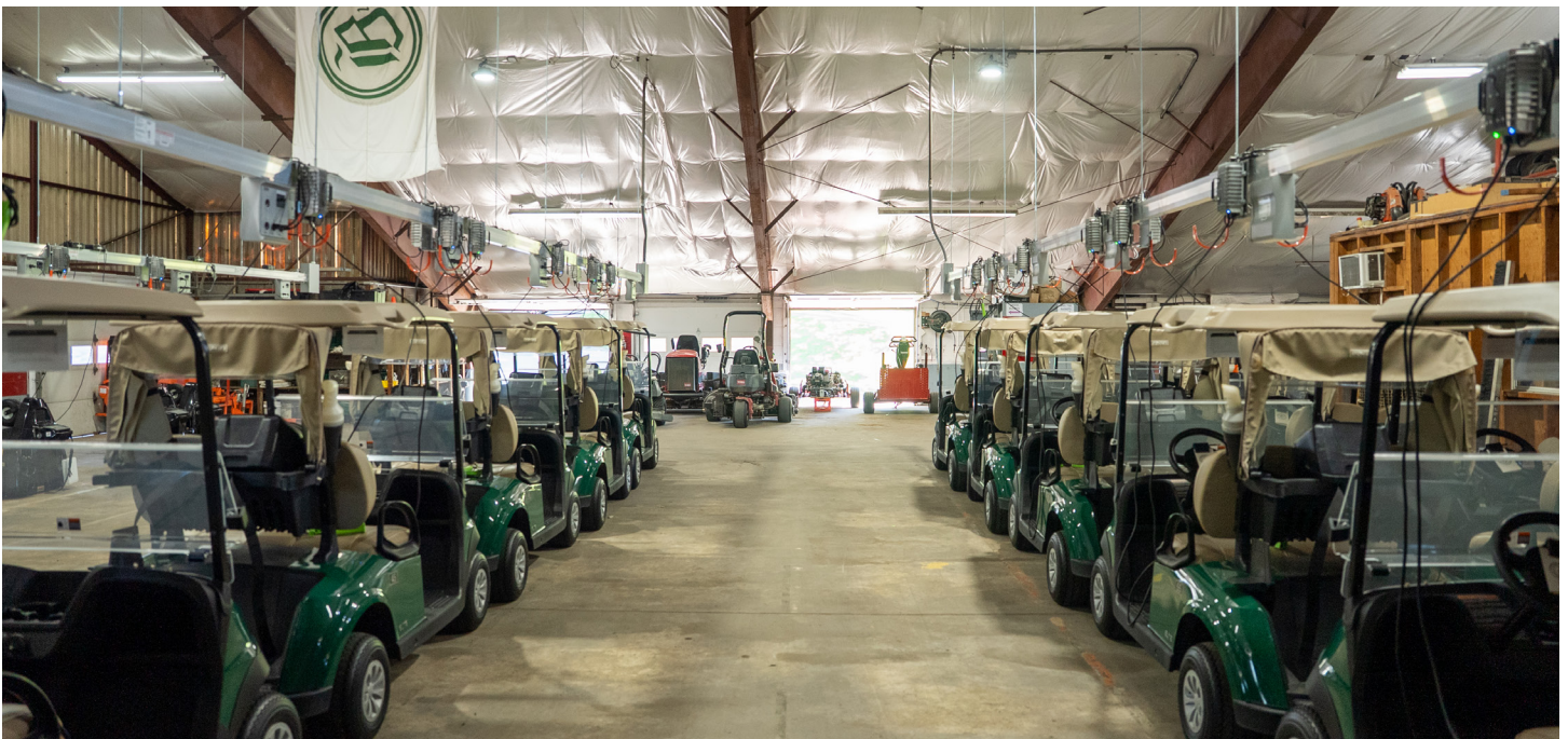
Butler Country Club has streamlined charging with the new busway layout.
