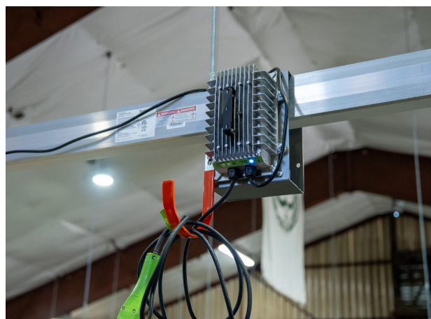
Custom brackets supporting the chargers are hung directly on the busway.
