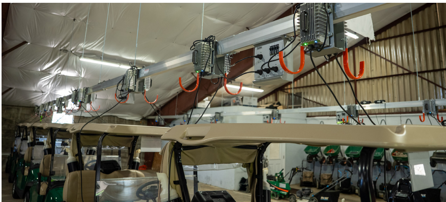
E-Z-GO chargers mounted on custom brackets sit directly above the carts.
