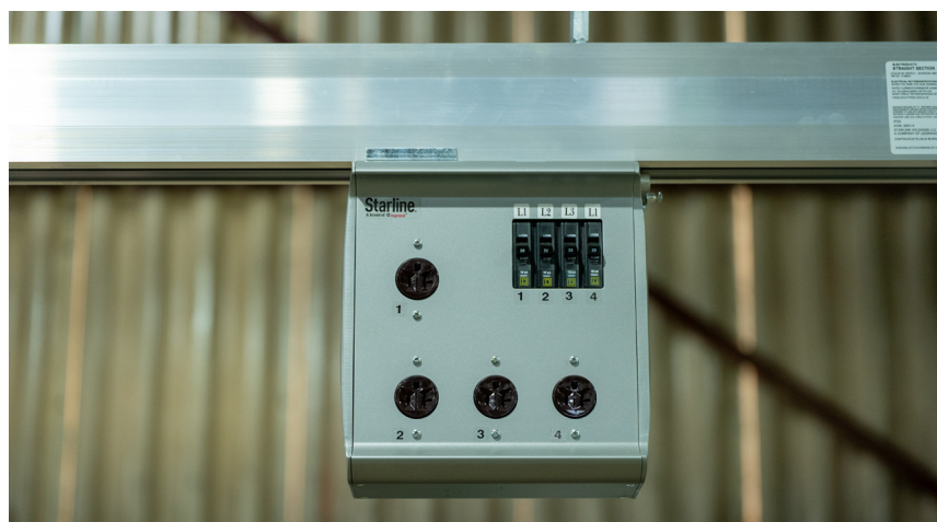
Plug-in unit inserted into busway housing.
