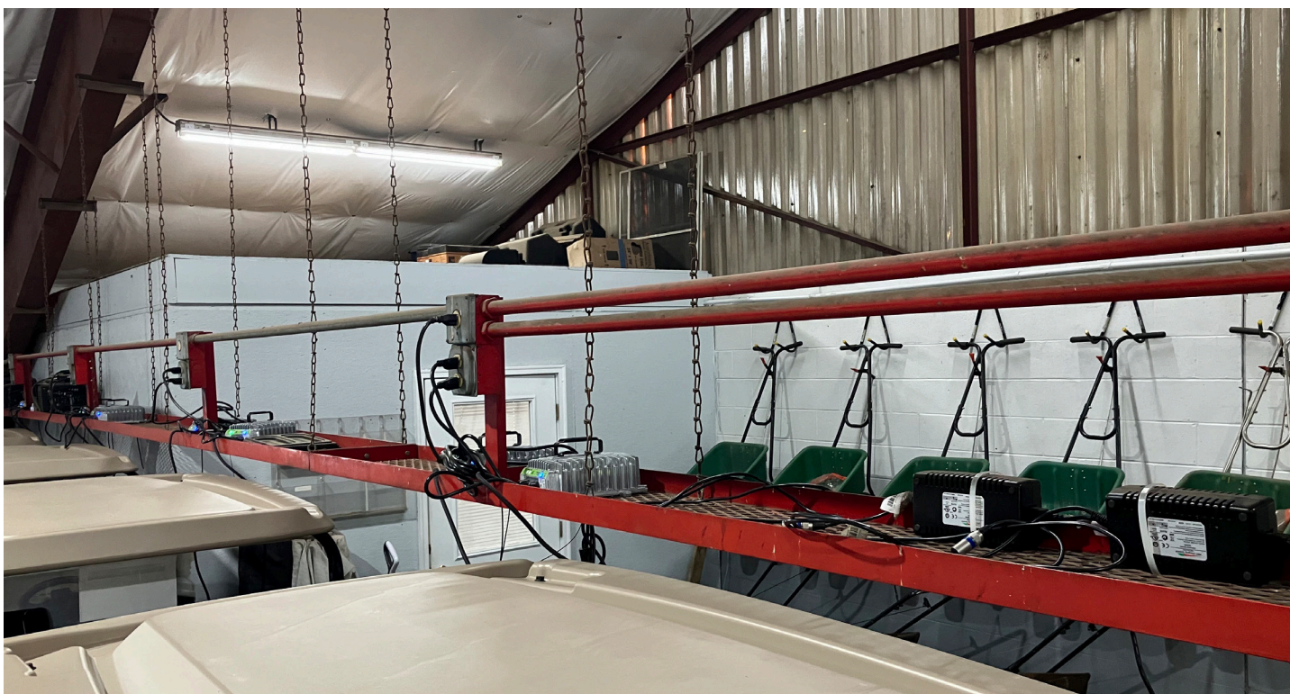
Butler's legacy charging system hung low and had limited outlets.
